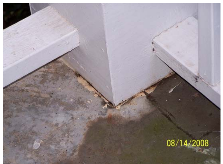
Seal at bottom of front porch posts
