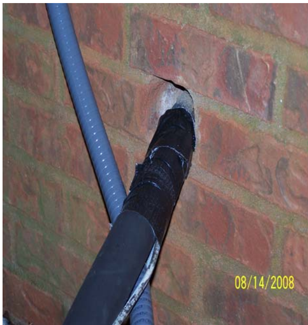
Seal hole around coolant lines
