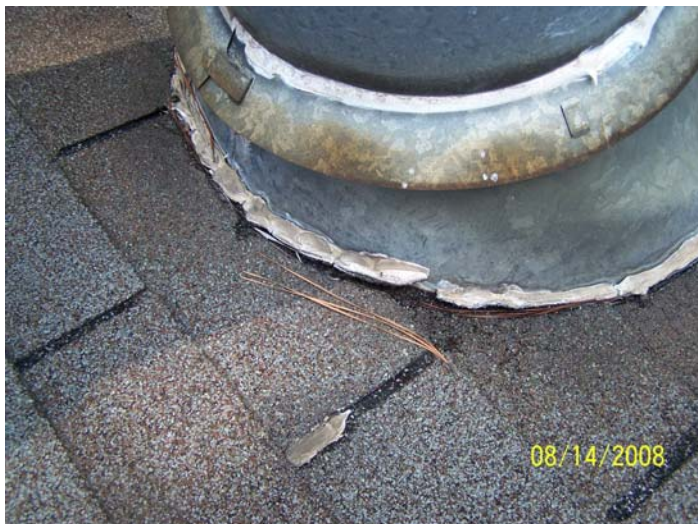
Replace caulking on chimney flashing
