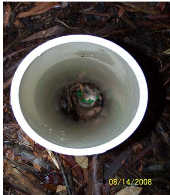
Main water shutoff
