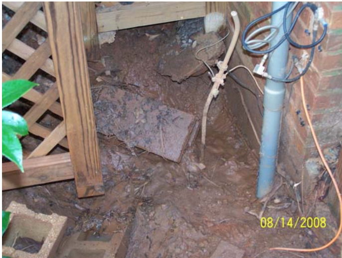
Eroded area in left rear
